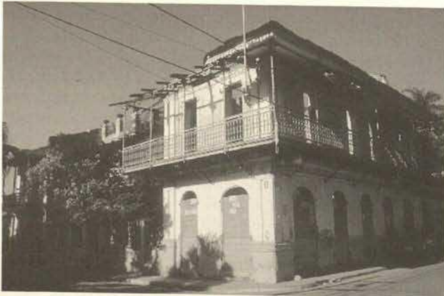
Damages caused by storms
